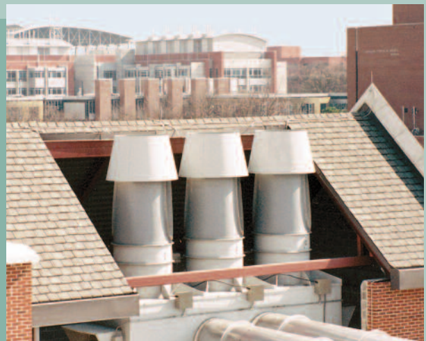
Duall Mixed Flow Exhausters with effective stack height of 60 feet.
