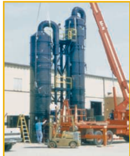
Application: Specialty steel production (acid etching) Problem: NO x and mixed acid fumes Solution: Beta NO x 2000® Two Stage
