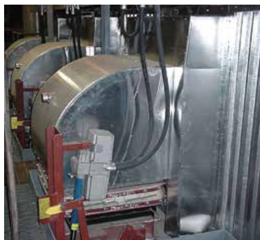
CCA's Overfire Air Ports
