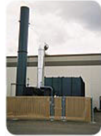
This 22,500 scfm dual-chamber RTO system provides greater than 99% VOC control of the styrene and alcohol HAPs for a Seattle-area manufacturer of windows and doors.
