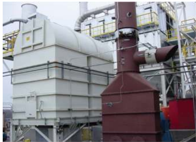
CECO Abatement 40,000 scfm RTO for ethanol VOC
