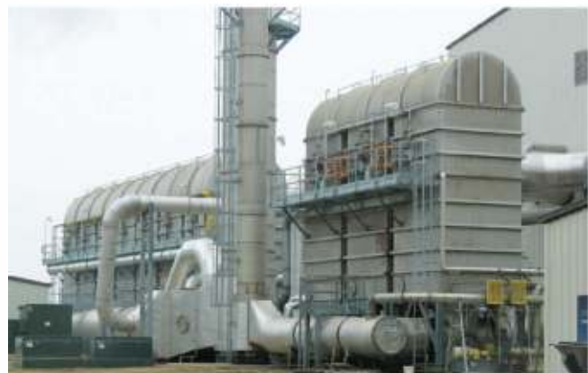
CECO Abatement 7 and 3 Bed RTO Oxidizers at Midwest Ethanol Plant
