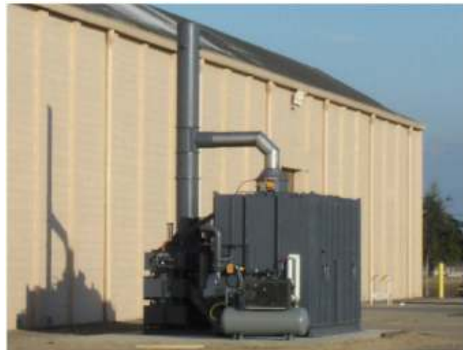
RETOX 5,000 scfm RTO for Wine and Brandy Ethanol VOC Control
