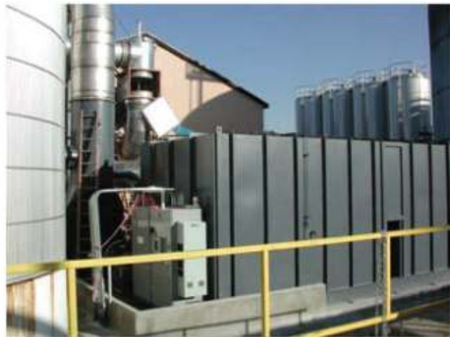
A dual chamber RTO oxidizer with 95% primary heat recovery.
