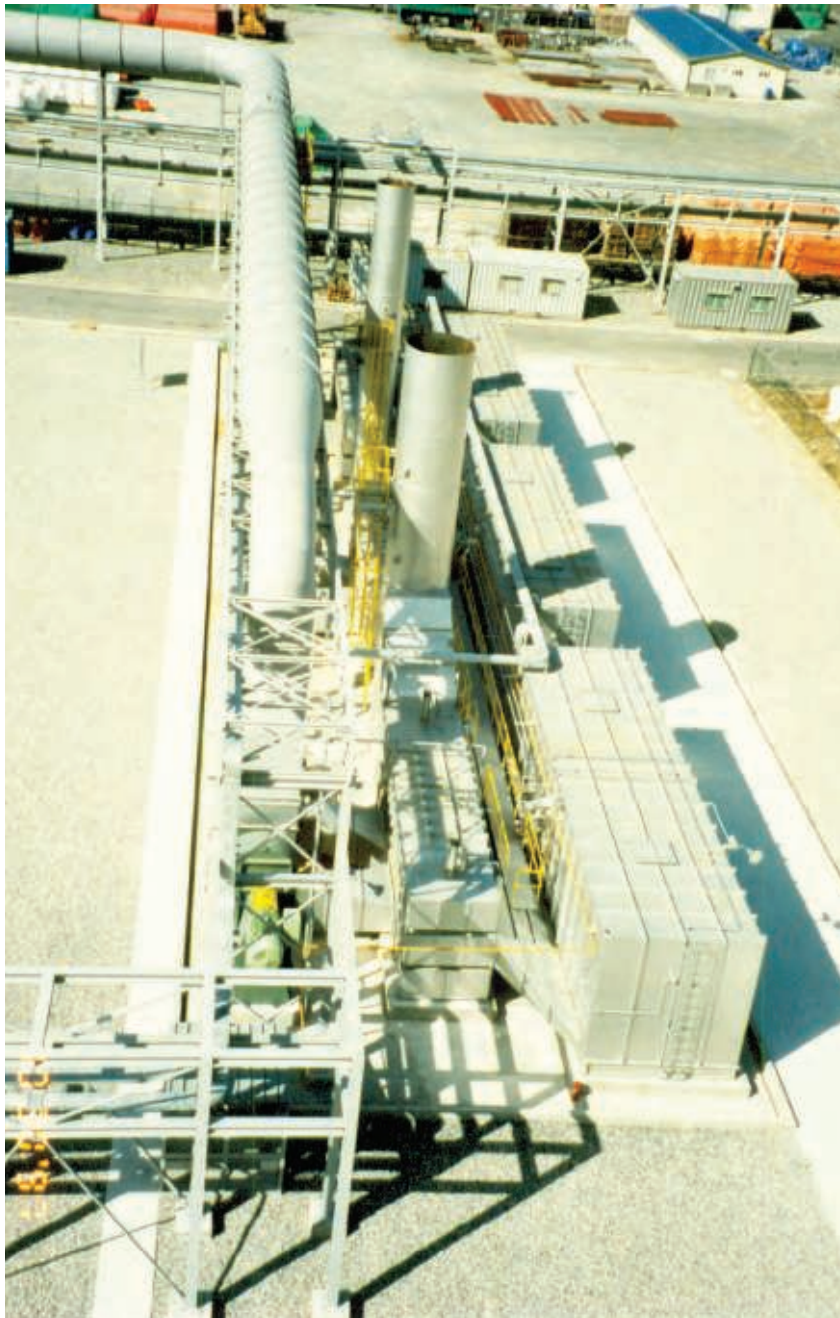
3 Module RETOX RTO System for 120,000 scfm Ethanol Chemical Processing
