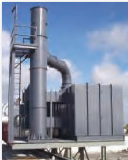
Rooftop/platform mounted Retox RTO for web offset printing.
