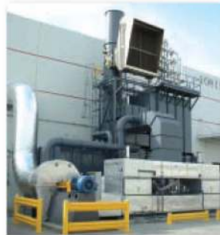
25,000 SCFM Retox RTO with secondary adsorption chiller.
