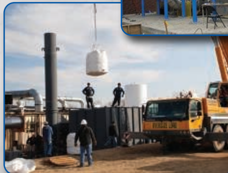
◀ RTO HX Media Upgrade
