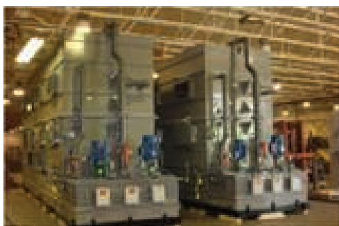
湿式洗涤塔 water scrubber
