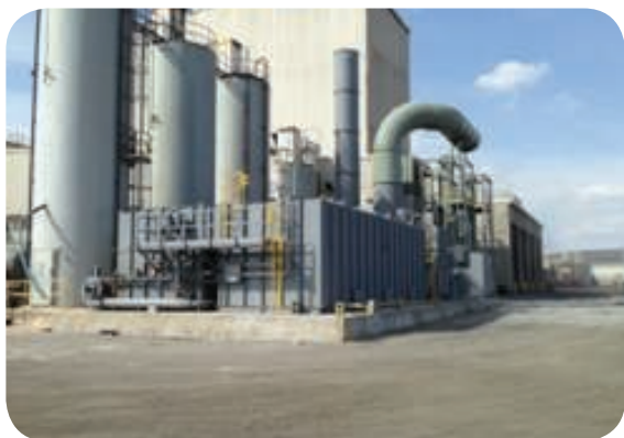
70,000 scfm RTO 处理铝铸造车间尾气 70,000 scfm RTO for Aluminum Foundry
