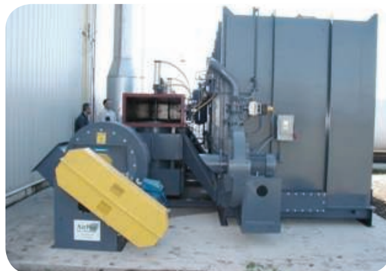
8000 scfm RTO 处理食品加工尾气 8000 scfm RTO for Food Processing
