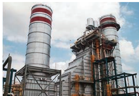
燃气轮机排气系统和消音设备 Gas Turbine Exhausting System & Silencer
