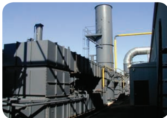
110,000 scfm RTO 处理汽车喷涂尾气 110,000 scfm RTO for Vehicle Spray
